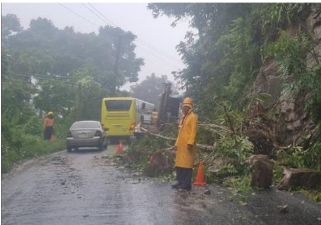
Figure 25: Massive rocks, soil and debris lying on the roadside due to the landslide on 27 th July, 2023 (Picture Credit: Fiji Roads Authority).
