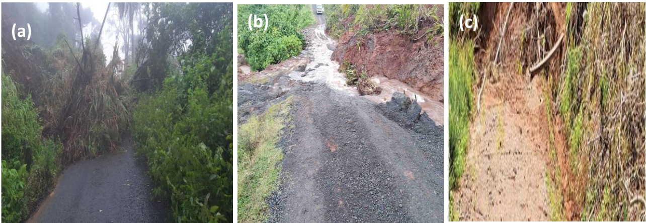
Figure 23: (a): Landslide in Nadarivatu on 18 th February, 2023 (Picture Credit: Fiji Roads Authority); (b) Landslide at Nakabuta settlement, Kubulau road, Wainunu, Bua on 21 st February, 2023 (Picture Credit: The Fiji Times); (c) Landslide in Paipai, Lautoka after heavy downpour on 23 rd February, 2023 (Picture Credit: Fiji Sun).
