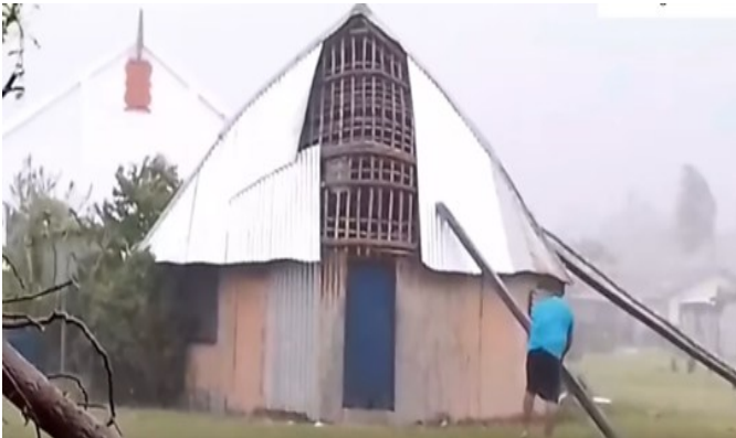
Figure 13g: Strong winds threaten to blow the roof off a home in Namuka-i-Lau on the 25th. Source: The Fiji Times.
