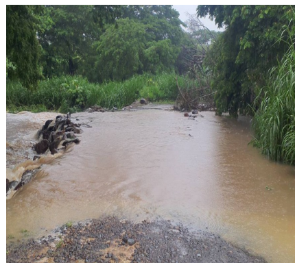
Figure 12c: Overflown Qalele Rd, Tavua. Source: Fiji Roads Authority.
